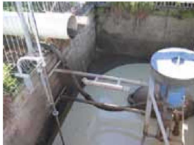
The solid contents of the biodigester flow out into a pit for use as fertiliser.
