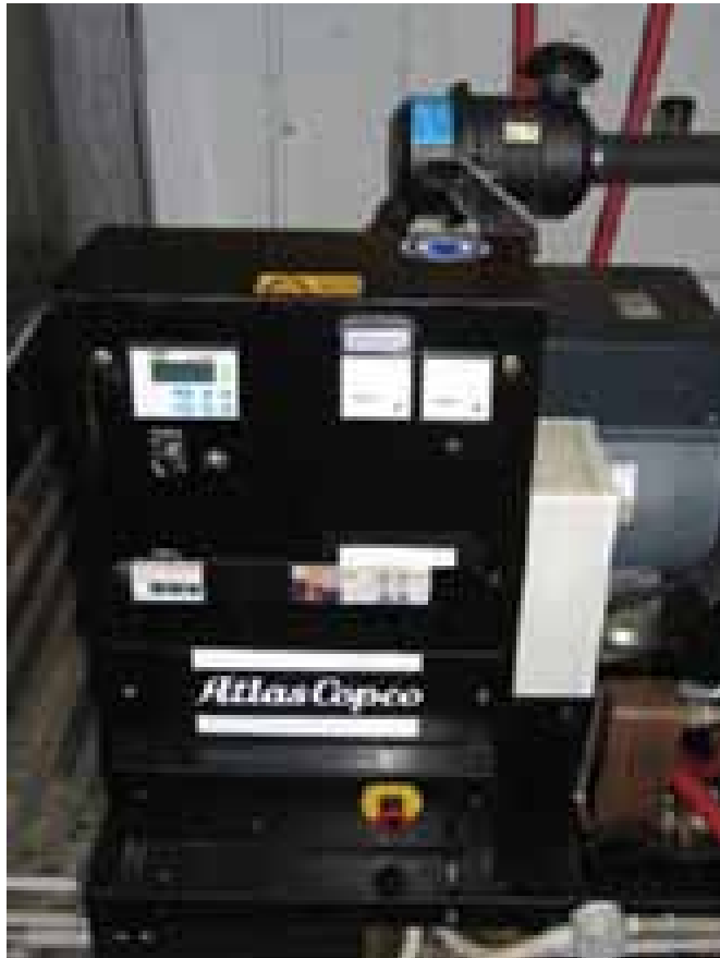
The generator uses biogas to generate electricity which is either used onsite or exported into the network.
